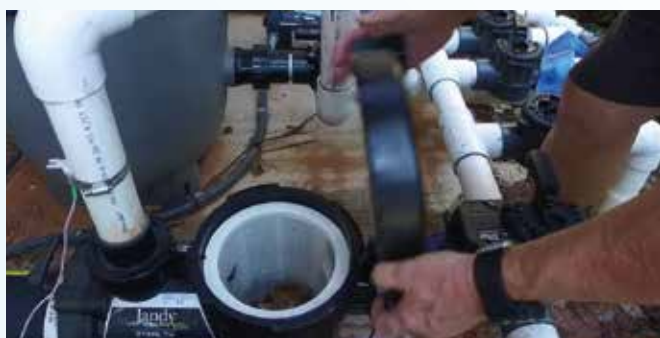
Circulation and filtration maintenance
